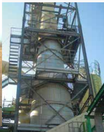
Fume cooling tower
